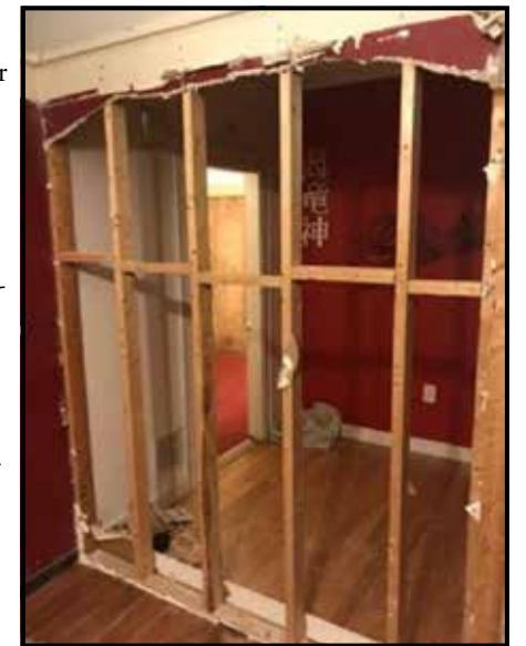
Converting Myles from a double to a triple by removing the wall separating it from the 4th hall closet.
